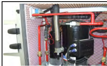
Compressor / Gas System
