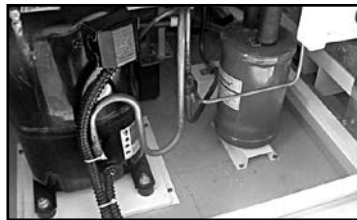
Compresor / Gas System
